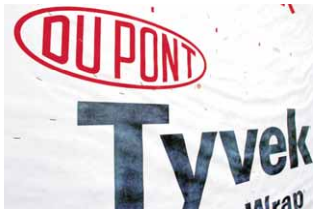
A DuPont logo on sheets of Tyvek insulation covering a wall of a home under construction in Springfield. — AP
