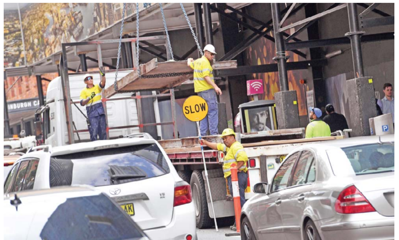
SYDNEY: Construction personnel work on a building site in central Sydney yesterday. Australia's economy contracted for just the fourth quarter in 25 years, official data showed, slowing the annual growth rate to 1.8 percent amid weaker government and consumer spending on top of softer trade figures. — AFP
