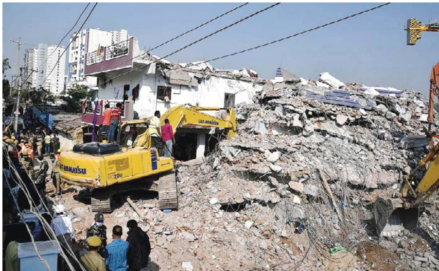
HYDERABAD: In this photograph taken on December 9, 2016, Indian rescue workers dig through the rubble of a collapsed building. — AFP
