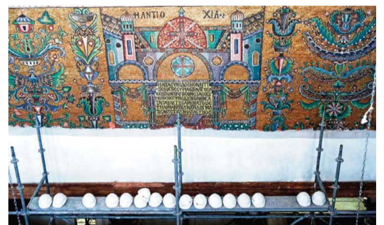
An ancient mosaic on a wall in the upper part of the Church of the Nativity, which was uncovered during restoration works by Italian experts at the site, in the biblical West Bank town of Bethlehem. — AFP photos
