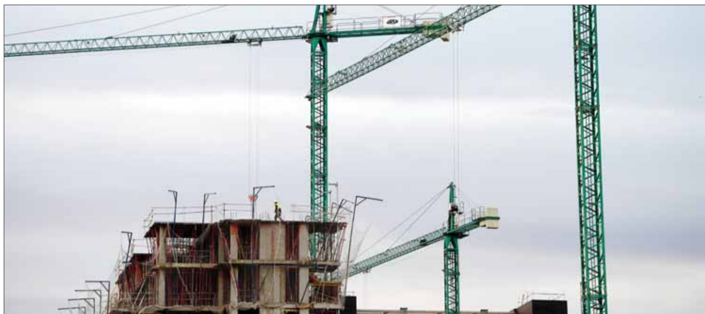
MADRID: A cranes seen at a construction site in Madrid. 2016 was poised to be a good year for Spanish builders but the lack of a government three months after an inconclusive general election has put the brakes on economic activity. — AFP
