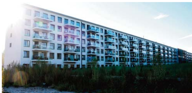
A construction site of luxury apartments as part of transformation of the heritage-protected Prora Complex.
