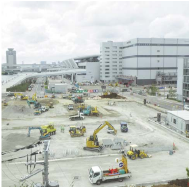
TOKYO: A construction site in Tokyo yesterday. Japan's economy barely grew in the April-June quarter, revised data showed yesterday, supplying the latest failing report card for the prime minister's policy blitz. —AFP
