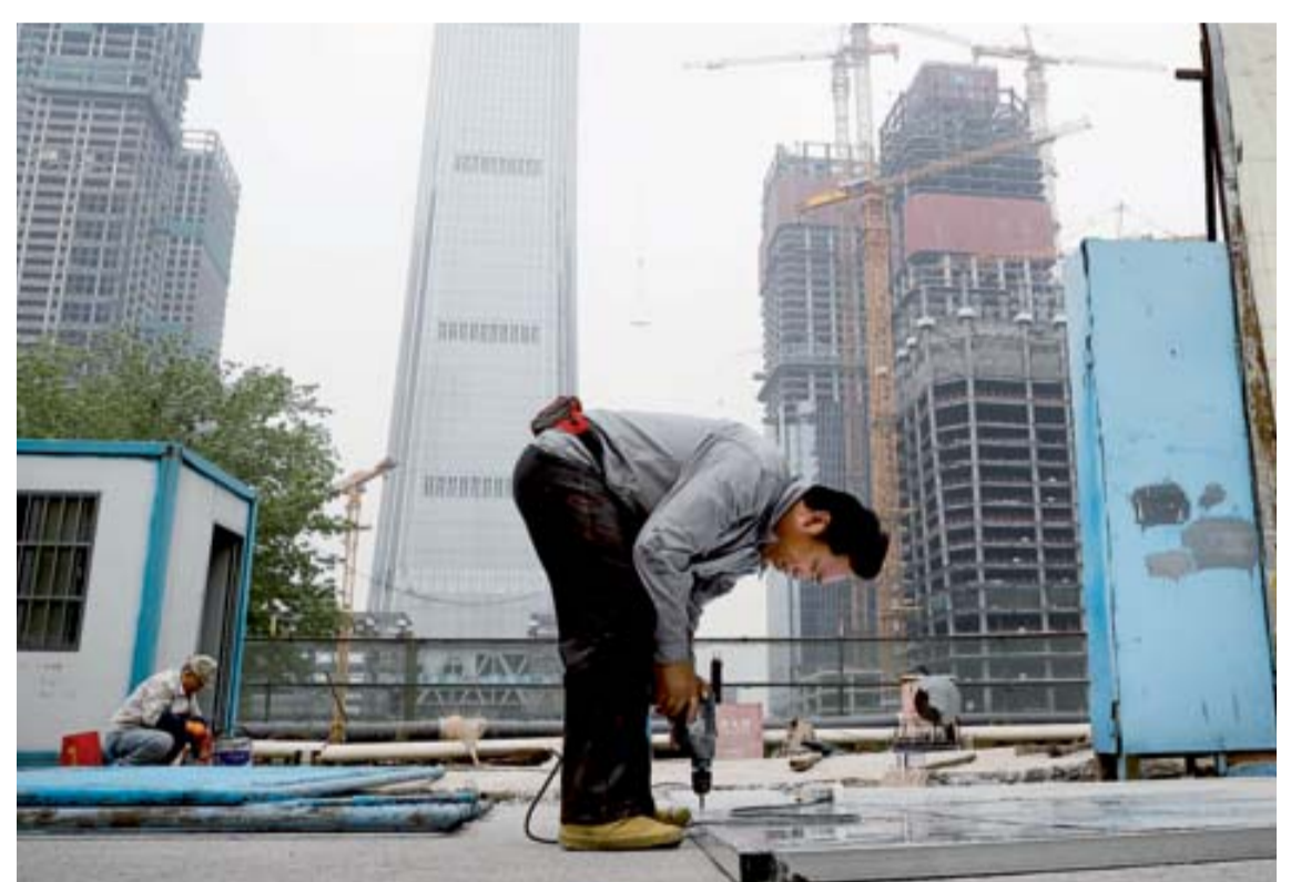
BEIJING: A worker assembles an aluminum platform outside a construction site at the Central Business District of Beijing. China's economic growth ticked higher to 6.9 percent in the first quarter of the year, according to the latest figures. —AP
