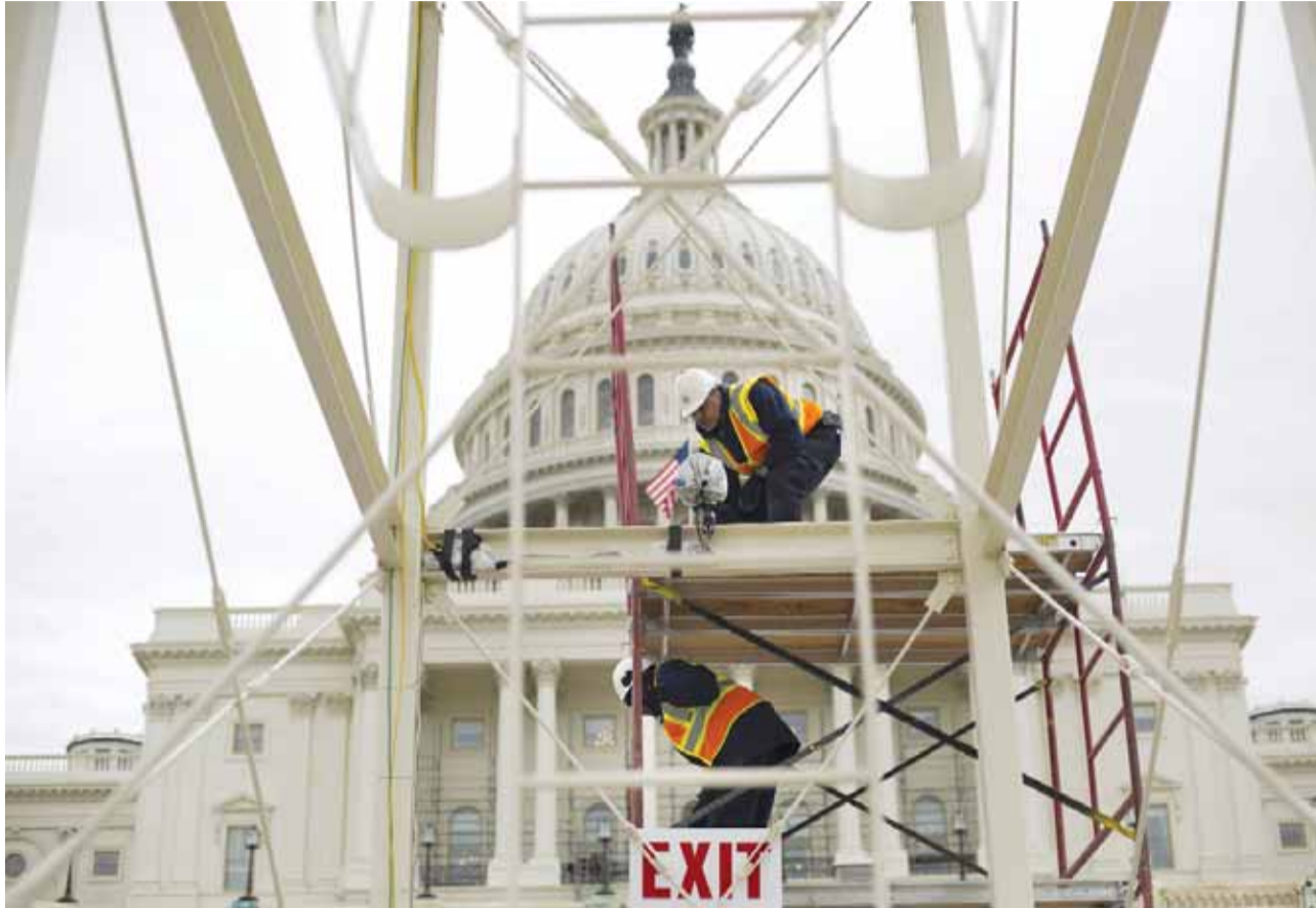
In this Dec 8, 2016 file photo, construction continues on the Inaugural platform in preparation for the Inauguration for President-elect Donald Trump on the Capitol steps in Washington, DC. Trump's Presidential Inaugural Committee has raised a record $90 million-plus in private donations, far more than President Barack Obama's two inaugural committees. — AP
