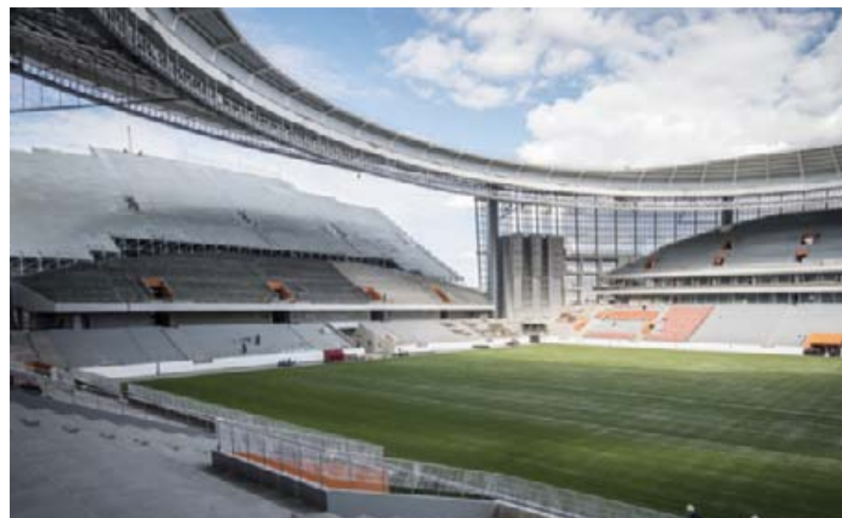
Yekaterinburg: A photo taken on August 19, 2017 shows the Yekaterinburg Arena football stadium under renovation work in Yekaterinburg. Football fans visiting Yekaterinburg in the Russian Urals for the 2018 World Cup will find out when they get seated in one of two temporary stands that fill empty plots of land next to the arena. — AFP
