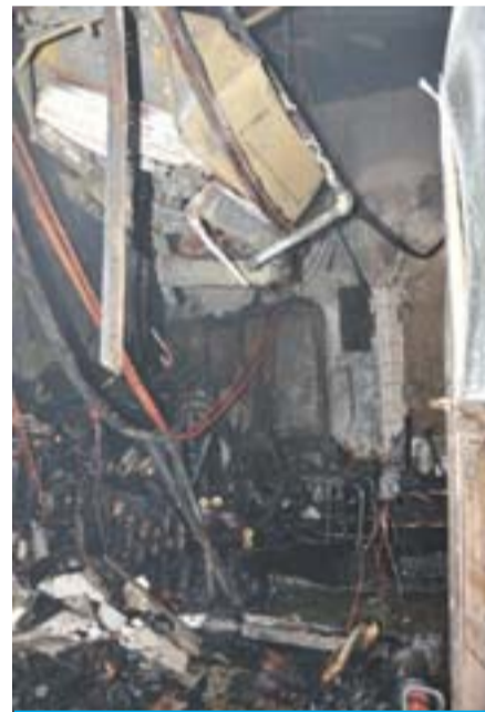
KUWAIT: Damage left by a fire reported in a Salmiya restaurant yesterday.
