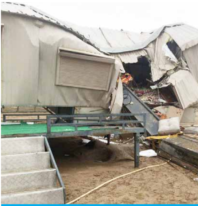
KUWAIT: A picture taken from the scene showing a heavily damaged chalet after a crane fell on it in Abdaly, killing a child and injuring three other family members.
