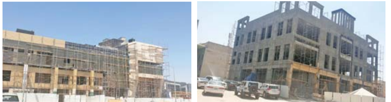
KUWAIT: A Kuwait Times tour in Jahra around 2:00 pm yesterday revealed that most construction projects were complying with the ban on outdoor labor during the day, contrary to what has been detected in sites located in other governorates around the country. — Photos by Ben Garcia
