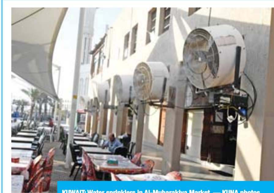
KUWAIT: Water sprinklers in Al-Mubarakiya Market. — KUNA photos
