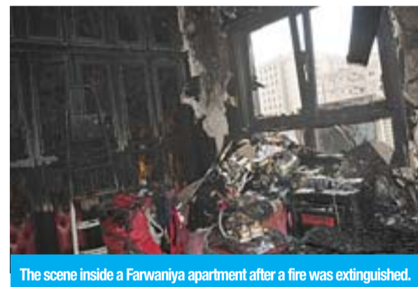
The scene inside a Farwaniya apartment after a fire was extinguished.
