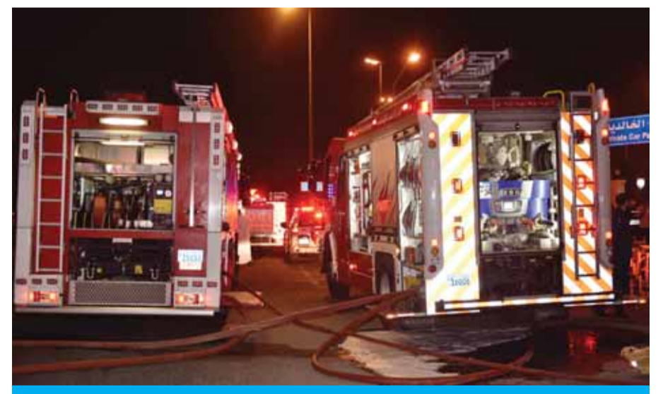
KUWAIT: A power transformer at Kuwait University's Khaldiya campus caught fire Sunday night. Industrial Shuwaikh and Shuhada fire station responded and put out the blaze. No injuries were reported. — By Hanan Al-Saadoun
