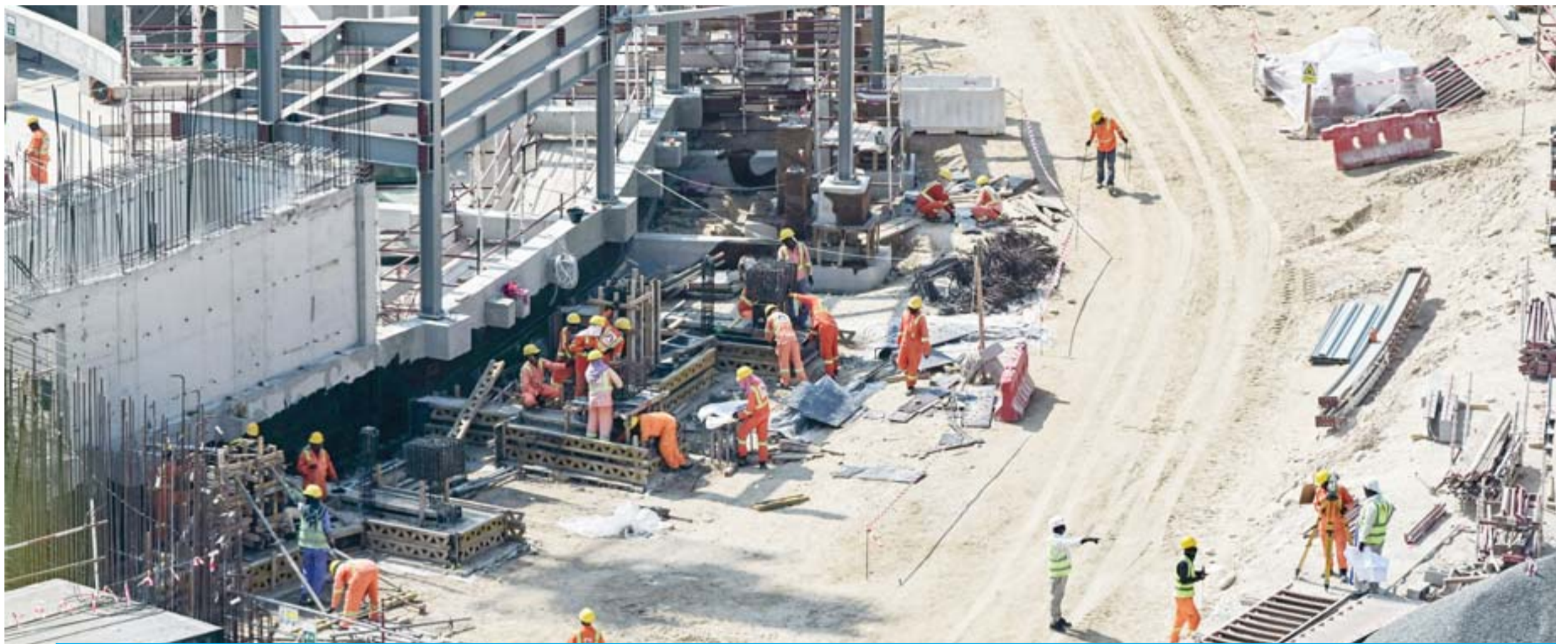
DUBAI: This picture taken yesterday in Dubai shows a view of ongoing construction work at the site of the Expo 2020, a big-budget global trade fair the glitzy emirate's rulers hope will restore its flagging fortunes. — AFP
