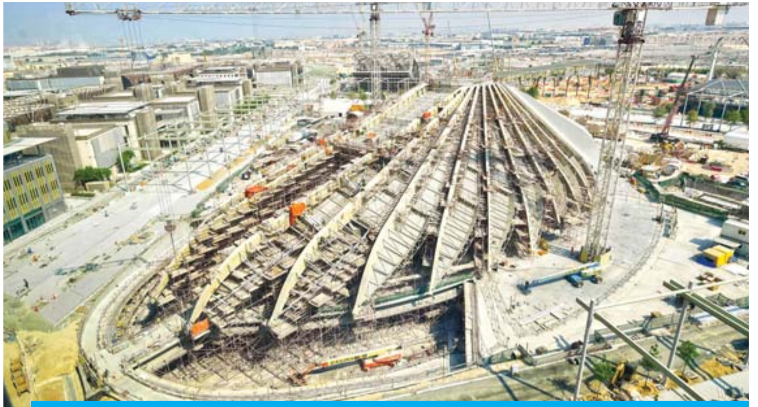
DUBAI: View of ongoing construction work yesterday at the site of the Expo 2020. — AFP
