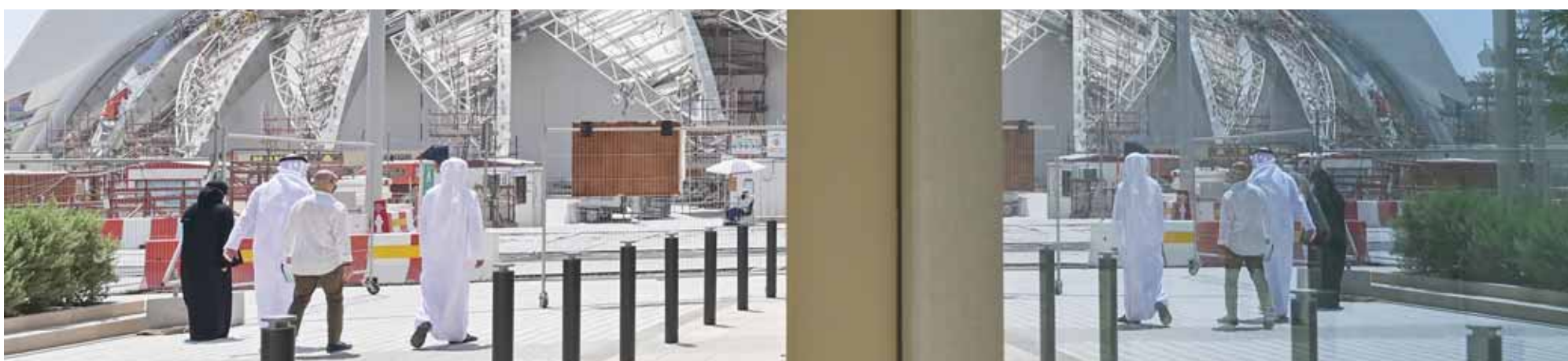
DUBAI: Emiratis visit the Dubai Expo 2020 site, under construction in the Emirati city. Armies of workers in protective masks are racing to complete the mammoth Dubai Expo 2020 site despite the coronavirus that has sickened some workers. —AFP
