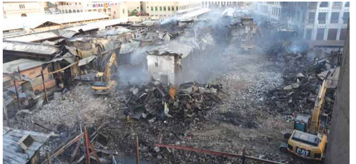
Photo taken on April 1, 2022 shows the damaged Souq Mubarakia after the fire.
