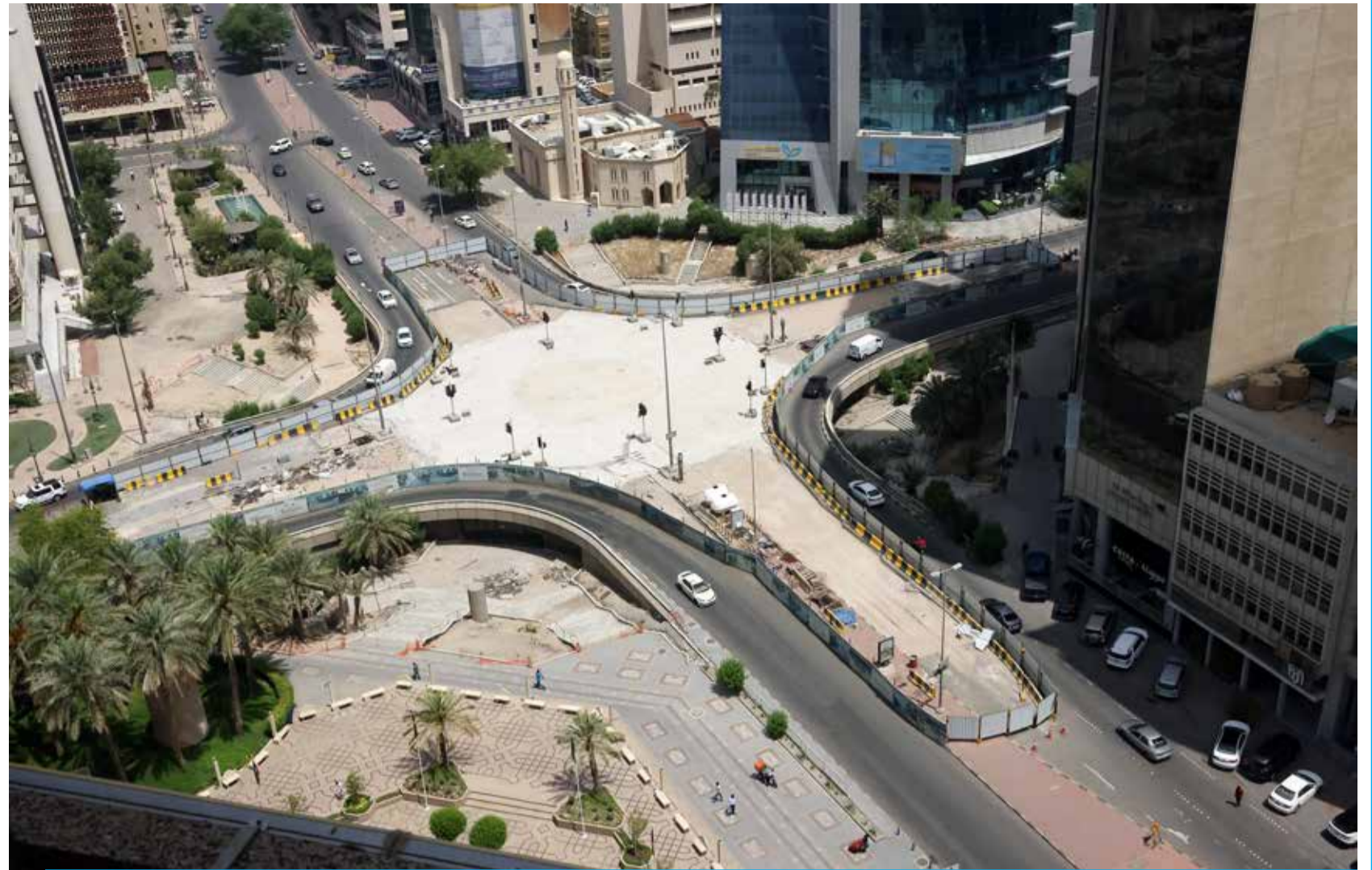
KUWAIT: This aerial photo shows the Darwaza Al-Abd Al-Razzaq tunnel and intersection in Kuwait City. The tunnel and intersection have been closed to traffic since October 2020 for a maintenance project. The project was set to be concluded in January 2023, following several delays. — Photo by Yasser Al-Zayyat
